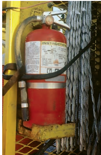
The fire extinguisher is easy to grab in an emergency.
