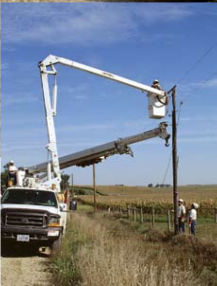
9 When the new pole was solidly in position, Armstrong "tied" the "hot" wire to the top insulator.
