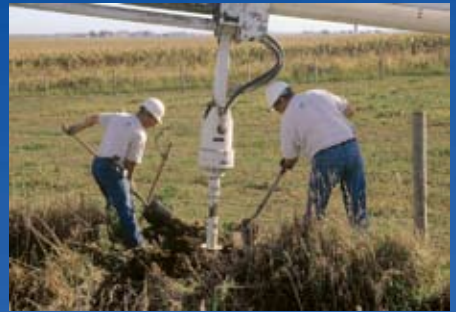
5 Weiland and Dolash cleared dirt from the auger as Armstrong bored the hole for the new utility pole with the digger derrick truck.
